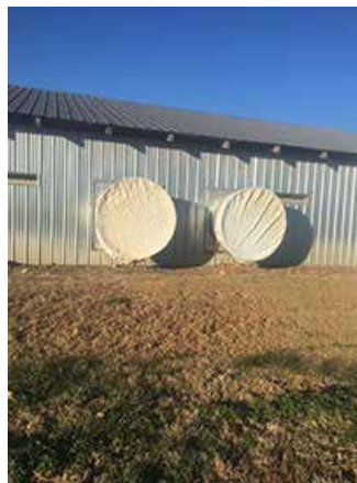
Figure 1. Tunnel fan covers help reduce air leaking around tunnel fan shutters.
