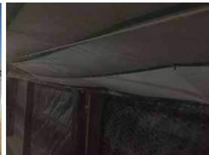
Figure 2. Wet insulation has a reduced effectiveness and can weigh down drop ceilings.
